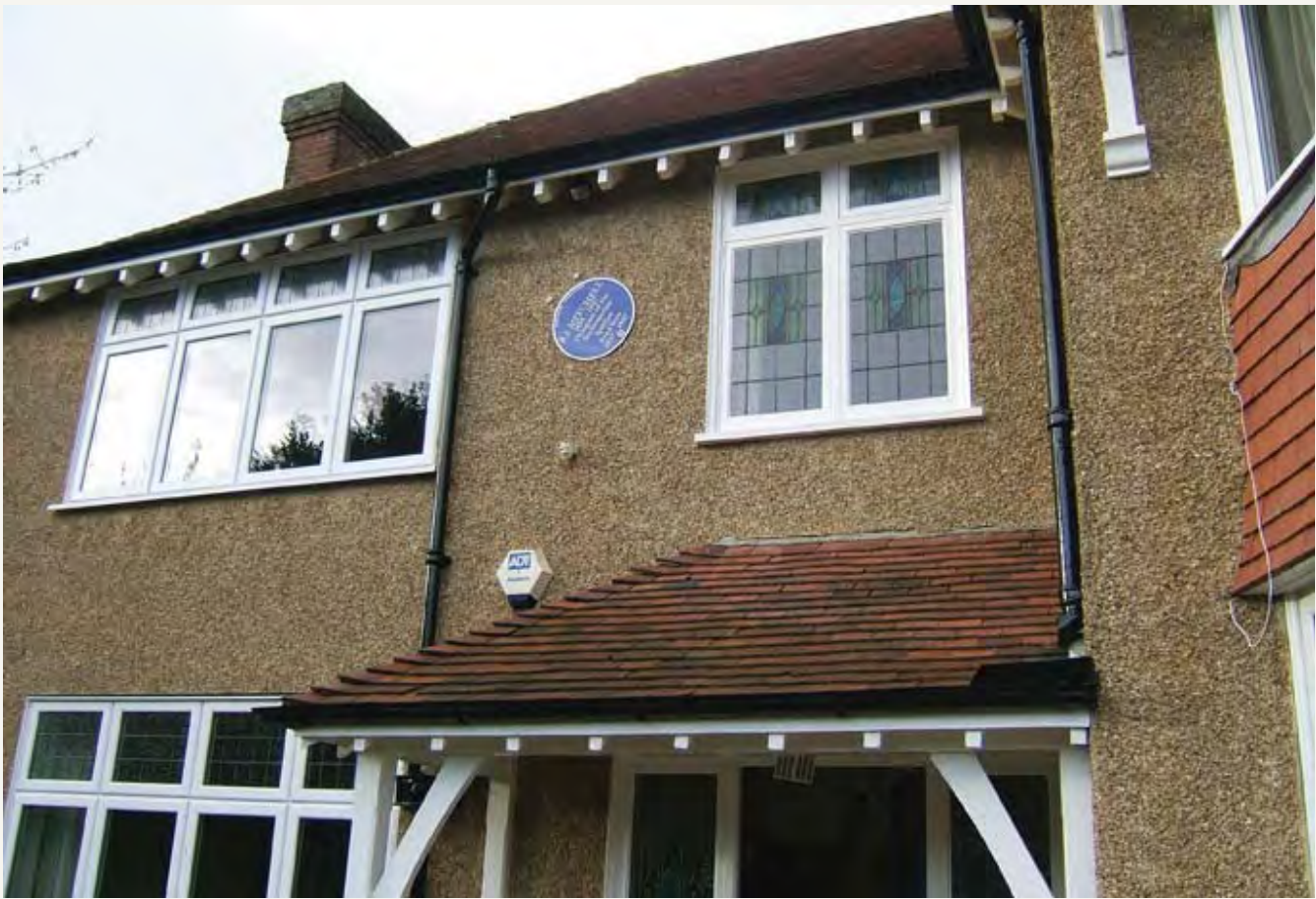
72 A photograph showing that disasters can occur with plaque manufacture and installation. This English Heritage plaque, commemorating R. J. Mitchell (1895-1937), designer of the Supermarine Spitfire, at 2 Russell Place, Portswood, Southampton, was made of enamelled steel. It had to be replaced after becoming partly detached from the wall three months after its unveiling in 2005.
