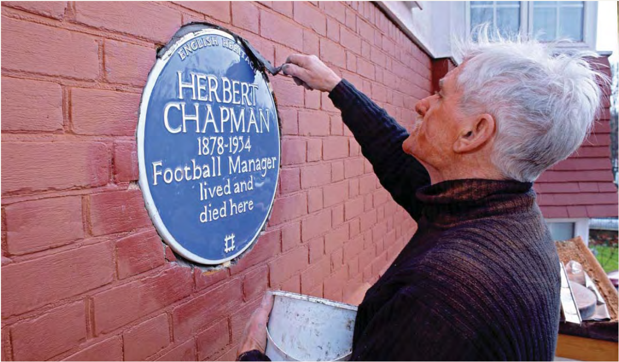
71 An English Heritage contractor installs the plaque to Herbert Chapman at 6 Haslemere Avenue, Hendon, London, in 2005. The installation of all plaques is a skilled job, especially those which need to be inset into the face of a wall.
