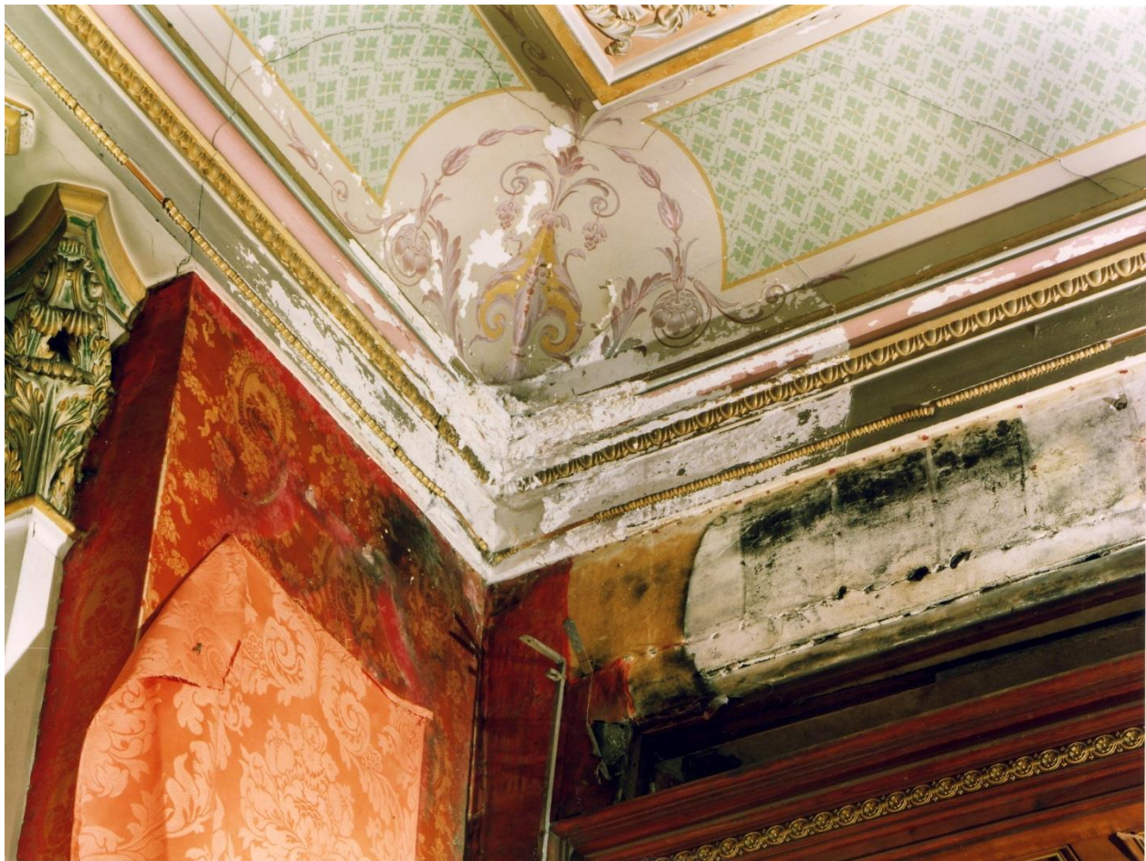
Fig. 6. Damage caused by water ingress. © English Heritage.
